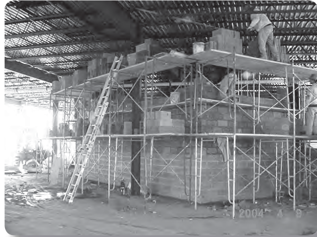
Problem: Conventional unguarded frame scaffolding
