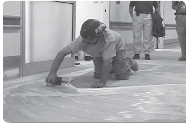
Problem: Kneeling to work near floor
