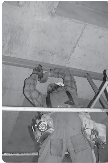
Problem: Using PAT overhead
