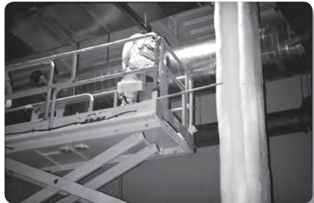
Person-lifts provide stable platforms for overhead work and eliminate handling of ladders and scaffolding
