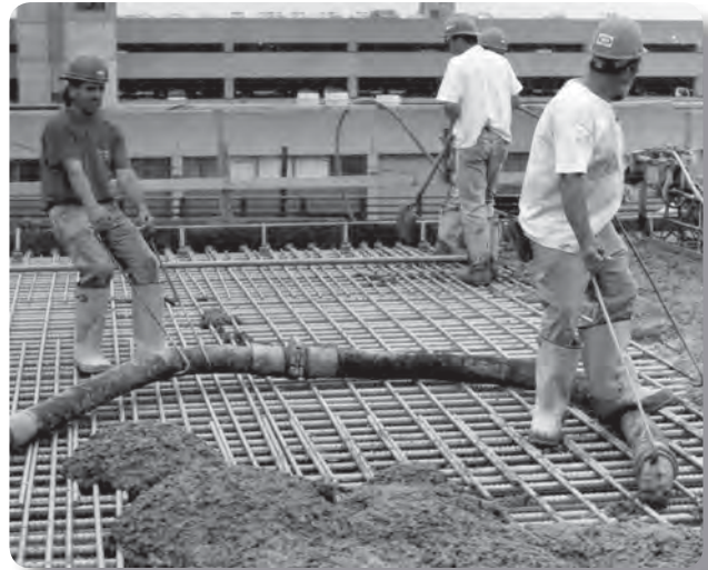
Problem: Pulling concrete hose without skid plate
