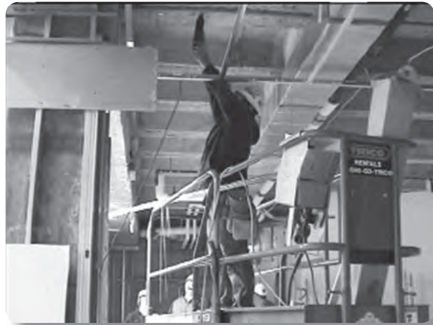
Problem: Drilling overhead
